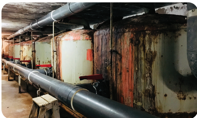
Corroded metal fabricated filters
