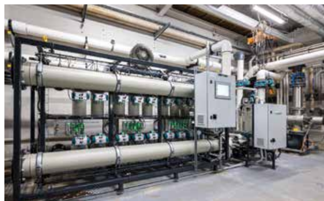
"The space saving design uses substantially less footprint, which is ideal when you have narrow access like we did or a plantroom with minimal room." Says Nick Yannakis, Powell Fenwick Technical Director.
