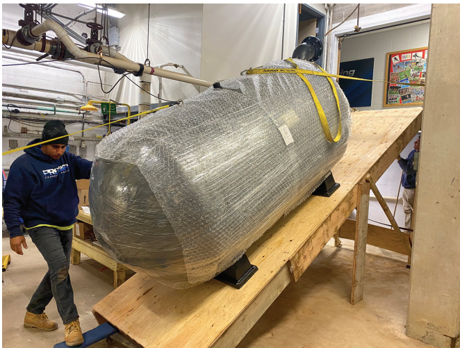
A ramp was built to position Waterco's Commercial Fiberglass Filters due to a narrow hallway into the equipment room.
