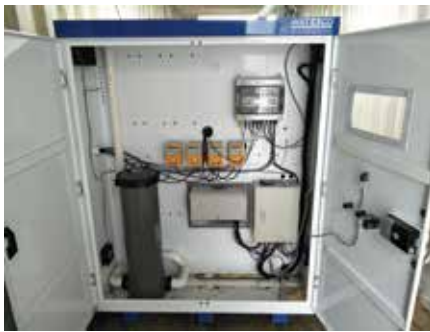
Waterco's Hydroxypure commercial system sanitising the 1.267 million litre Underwater dive tank.
