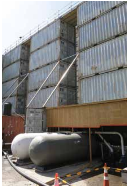
Ocean Surface Tank's external wall and its Micron M5000 horizontal filters.
